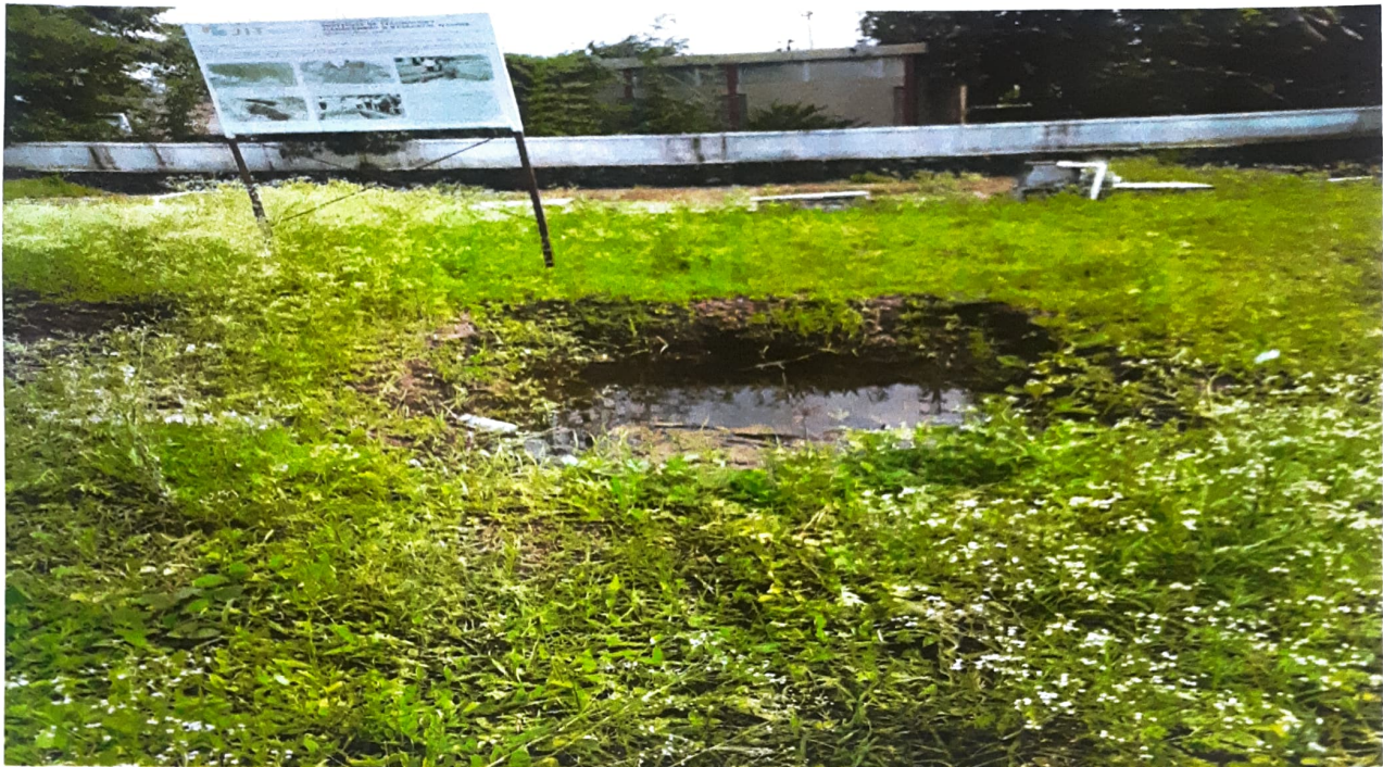
SEWAGE COLLECTION SOAK PIT
