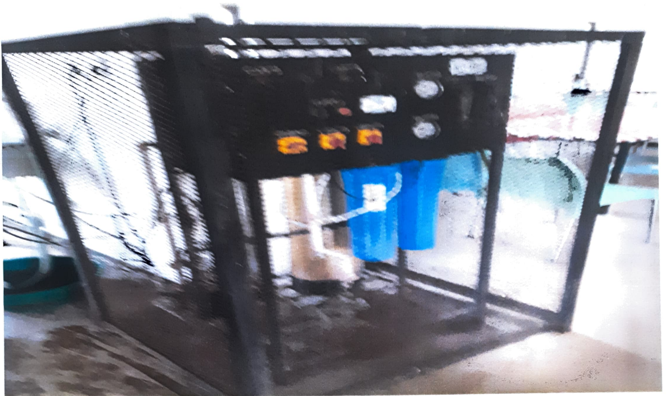
RO UNIT FOR DRINKING WATER
